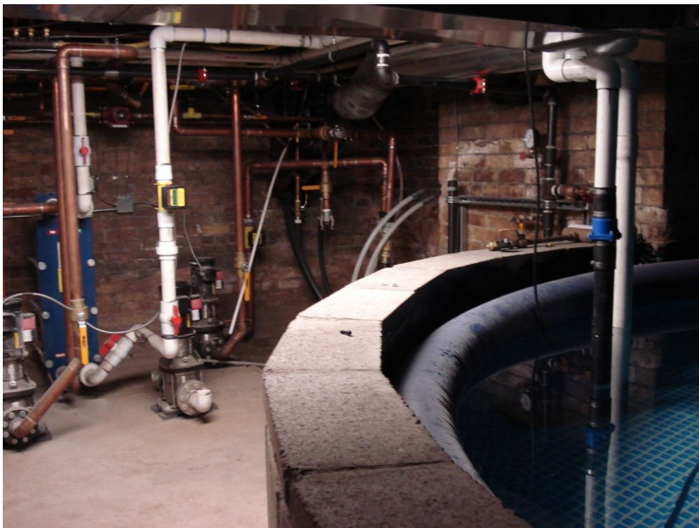
Figure 4: Mechanical room and interior water tank
