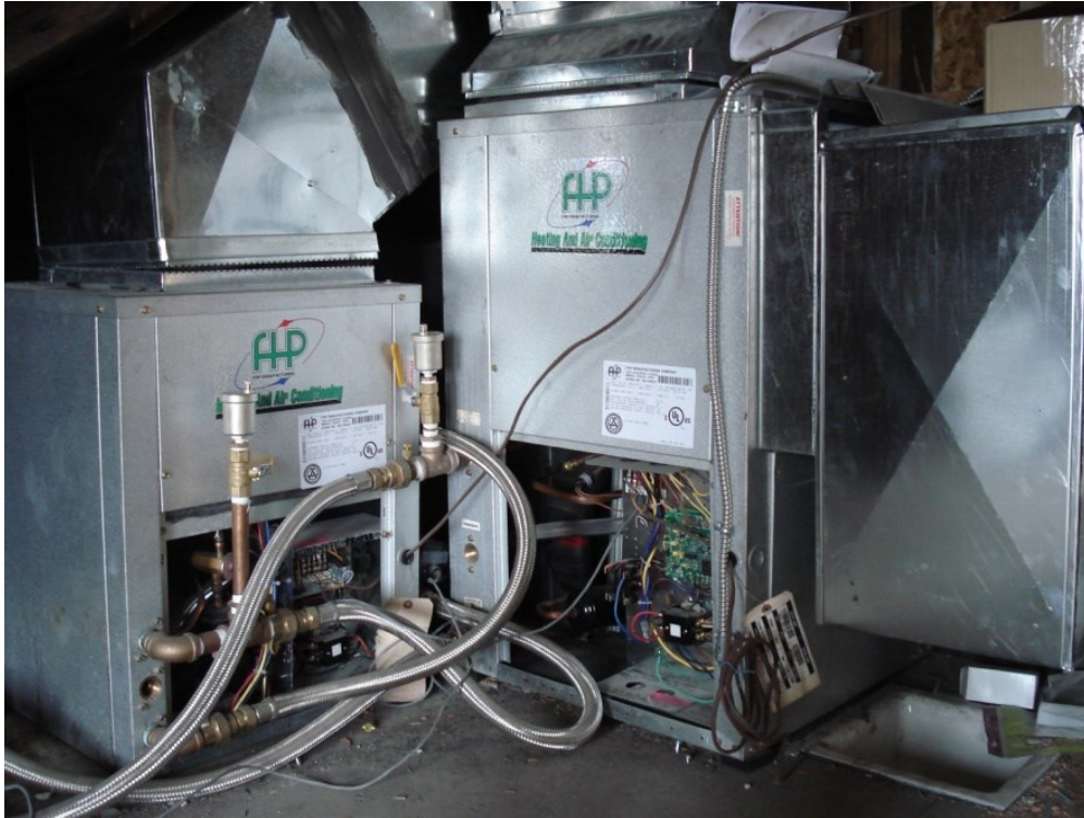
Figure 3: Heat pumps on third floor
