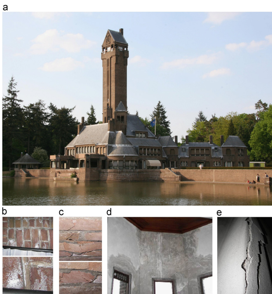
Figure 9 (a) Hunting Lodge St. Hubertus and moisture damage at the tower due to wind-driven rain; (b) salt efflorescence; (c) cracking/blistering due to salt crystallisation; (d) rain penetration and discolouration; (e) cracking at inside surface ( Briggen et al., 2009 ).
