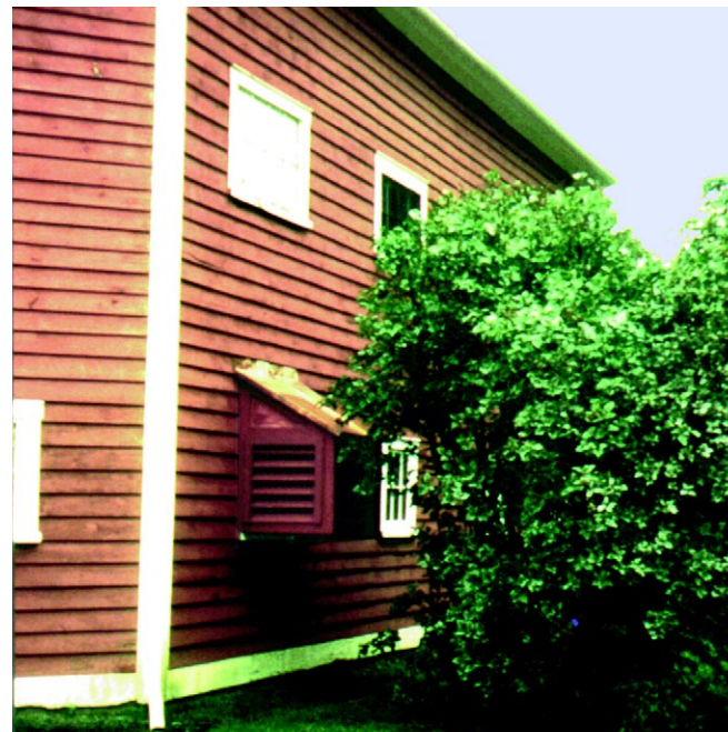
Figure 3: The Shelburne Museum, an outdoor art and history museum in Vermont, uses well-disguised ventilation fans with dust filters. The fans are controlled by humidistats to cool and lower humidity in buildings during warm weather. Increased air motion helps control mold growth. During the winter when the museum is closed, temperatures are lowered substantially to increase beneficial relative humidity. Humidistatically controlled heating is used to reduce humidity in buildings during cool wet spring and fall weather.
