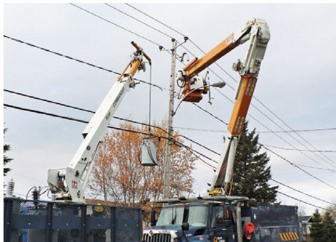
Fig. 5.9-1: Pole mounted, Canada
