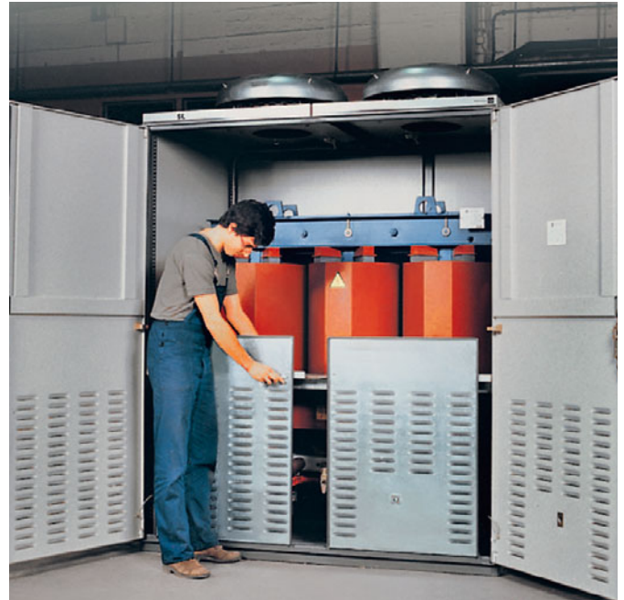
Fig. 5.9-9: GEAFOLE transformer in protective housing to IP20/40
