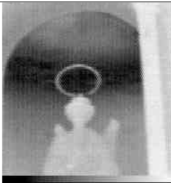
Fig 7: S.ta Maria in Cantuello, Ricengo (Cremona): passive thermography reveals a colder strip (40 cm large) behind the Angel Statue, 2.50 m up to the floor. A sod overgrown with moss coats the roof of the little niche and it is responsible of the infiltration.
